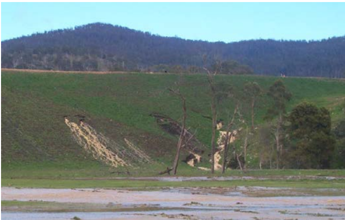
Figure 11. Seepage through the Embankment at Blackmon Dam in Tasmania
