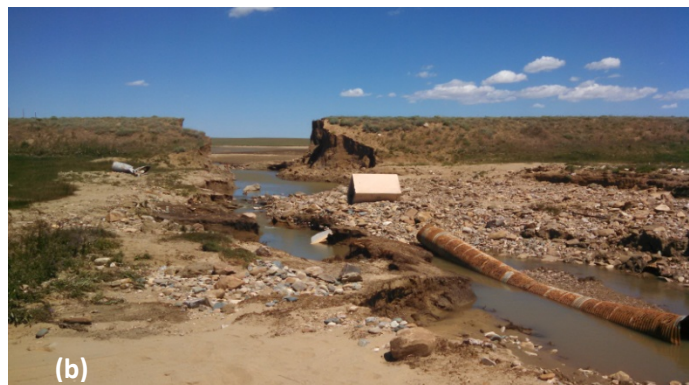
Figure 3. (a) Corrosion of a 40-year-old outlet pipe and (b) its effects.
