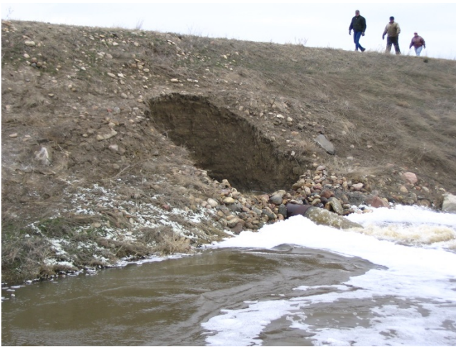
Figure 6. The Result of Concentrated Leak Erosion along a Conduit at a Dam in Montana
