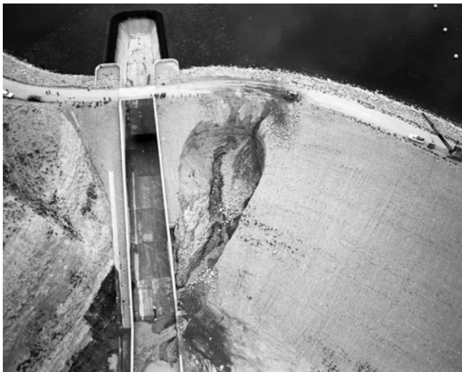
Figure 15. Partial Failure of Fontenelle Dam Due to Internal Erosion into Untreated Fractures in the Foundation [5]
