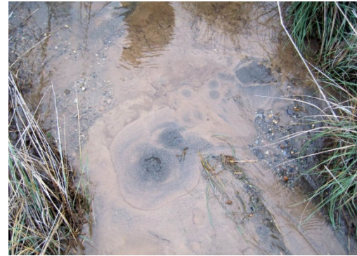
Figure 2. Sand Boil at Downstream Toe of Earth Dam
