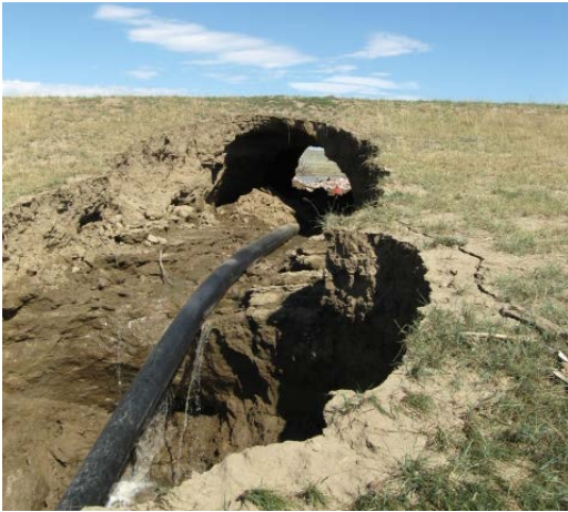
Figure 5. The Result of an Unfiltered Penetration through an Earth Dam in Wyoming
