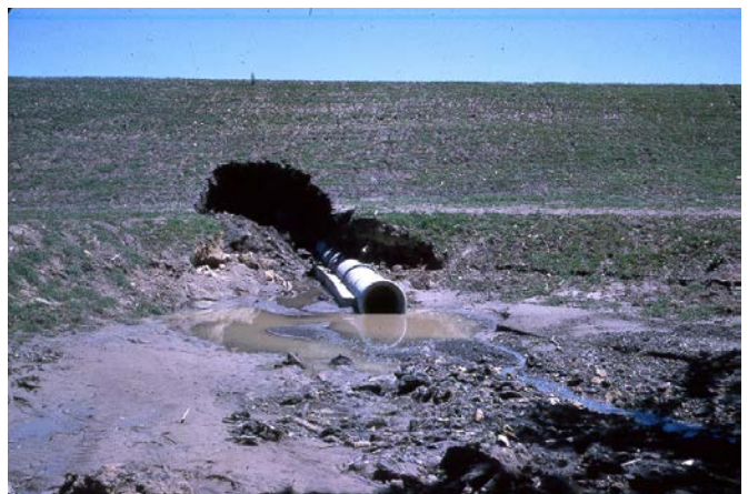
Figure 17. Internal Erosion along Conduits is a Common Failure Mode for Dams prior to the Use of Filter Diaphragms [1]
