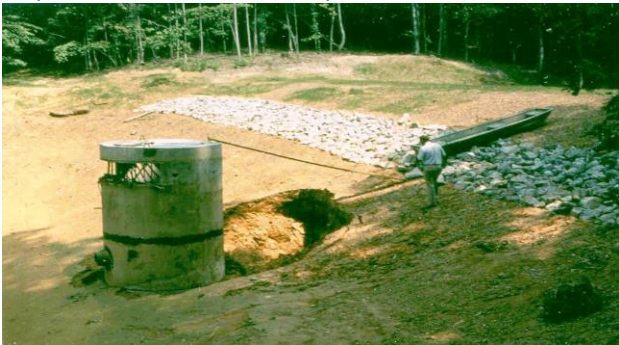
Photo 1: Sinkhole around a spillway riser 2
