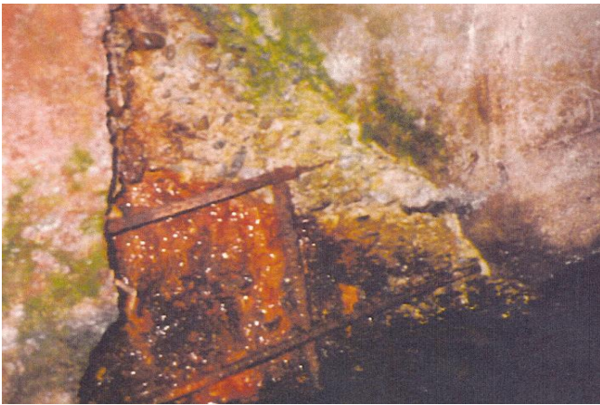
Photo 4: Spalled concrete inside a conduit. 2
