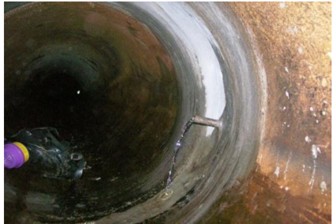
Photo 6: Grouted joint offset with grout port installed for injection grouting behind conduit.
