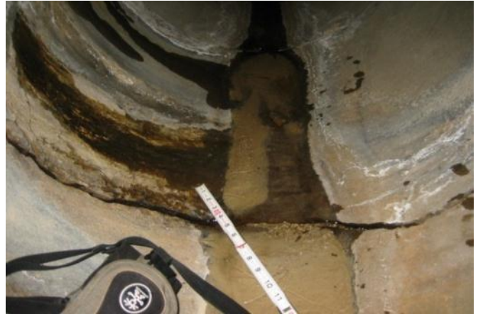
Photo 5: Crack in precast concrete conduit.
