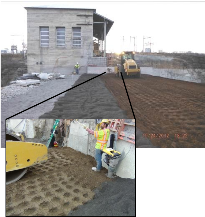
Photo 2. Core Compaction. Note compacting in paths parallel to dam axis and the hand tamper in photo that will be used to compact zone immediately next to wall.
