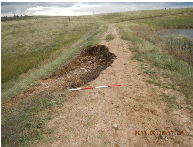
Photo 3. Slope failure on downstream slope
