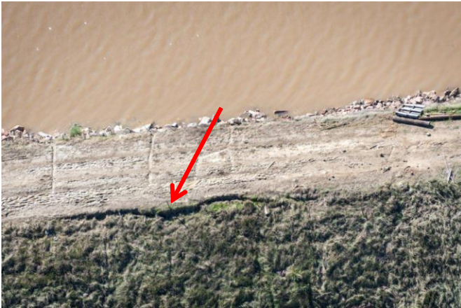
Photo 1. Severe longitudinal cracks in downstream slope
