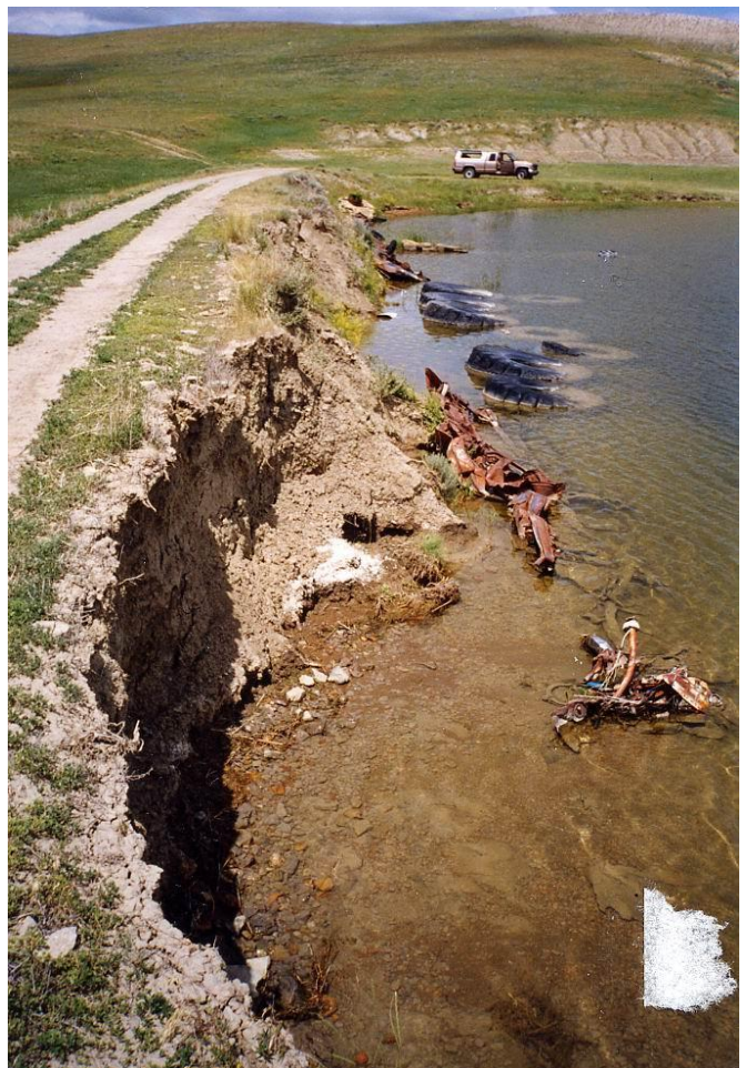
Figure 2: Erosion of a small embankment dam in Montana caused by wave action.
