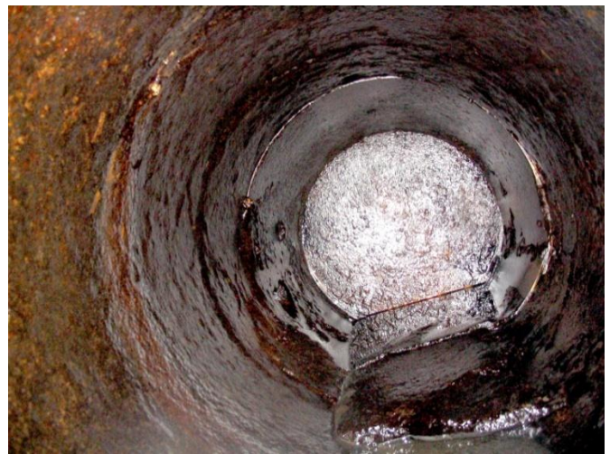
Figure 1: Typical cavitation damage on gate and conduit
