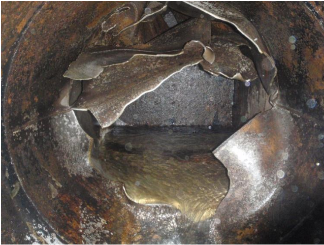
Figure 2: Outlet pipe liner collapse due to cavitation
