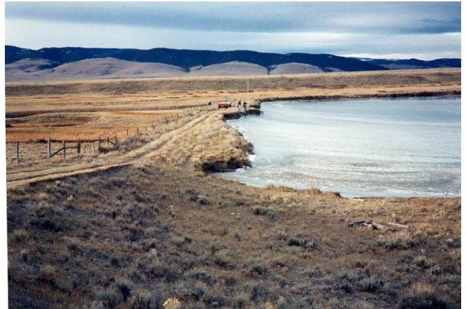
Figure 1: Erosion of a small embankment dam in Montana caused by wave action.
