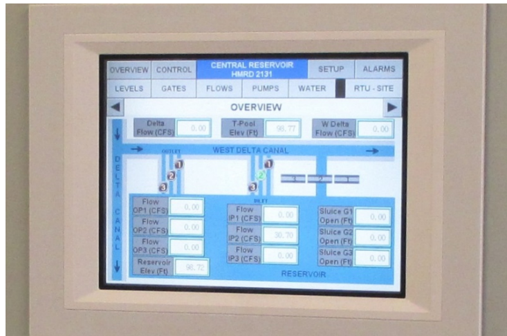
Figure 14. 12 inch touch screen example at San Luis Canal Company
