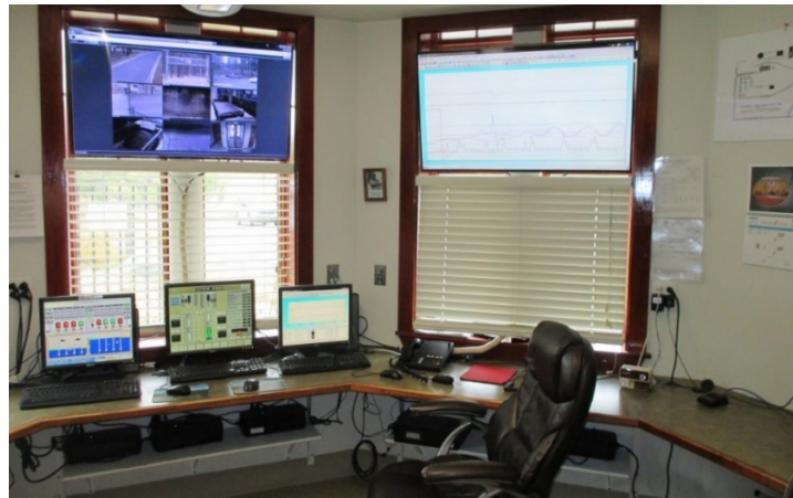
Figure 18. Base station example with multiple HMI screens and security camera
