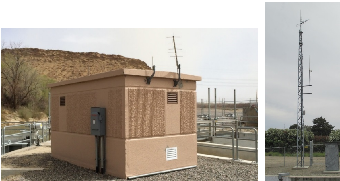
Figure 16. Large directional antenna mounted outside of a SCADA control building at Shiprock Irrigation District (left) and large antenna tower with multiple types of antennae at San Luis Canal Company
