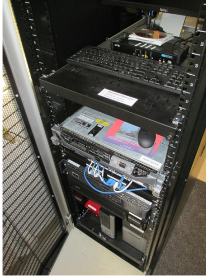
Figure 17. Medium-sized SCADA server rack with IT-related equipment
