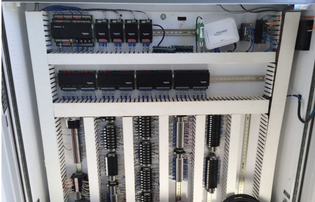
Figure 13. RTU cabinet internals example
