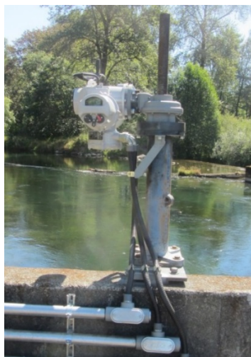
Figure 15. Rotork actuator retrofitted to a large, older sluice gate at Santiam Water Control District
