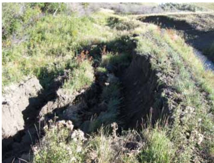
Erosion Issues Along Ditch Bank
