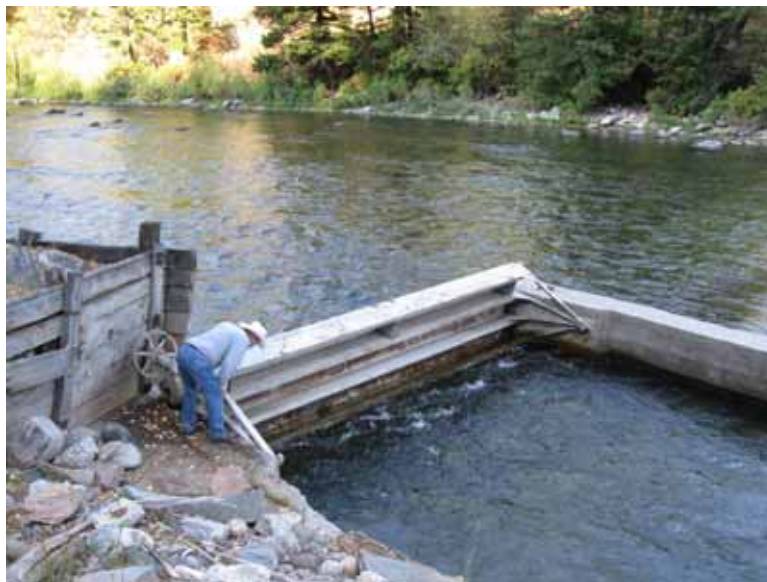
West Gallatin Canal Radial Gate at Diversion
