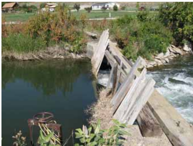
Benner's Check structure used to get water into distribution ditch headgate that can be seen in foreground of the photo.
