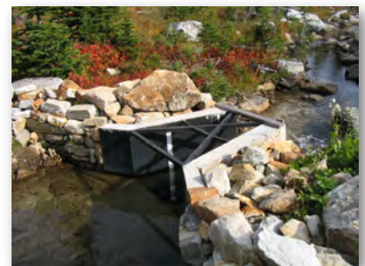
Parshall Flume installed below Mill Lake Dam.
